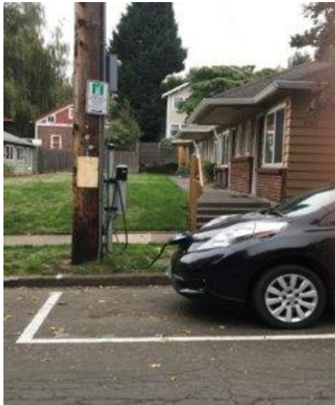
Pole charging pilot with Portland General Electric since 2020
